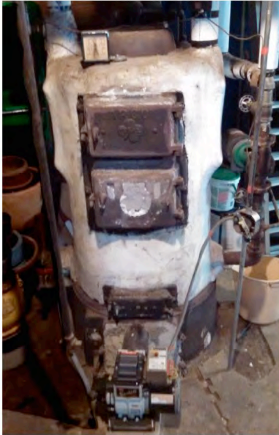
Boiler wrapped in asbestos insulation Picture from Expanded HEAT Loan Initiative Report , December 2015, E4theFuture.
